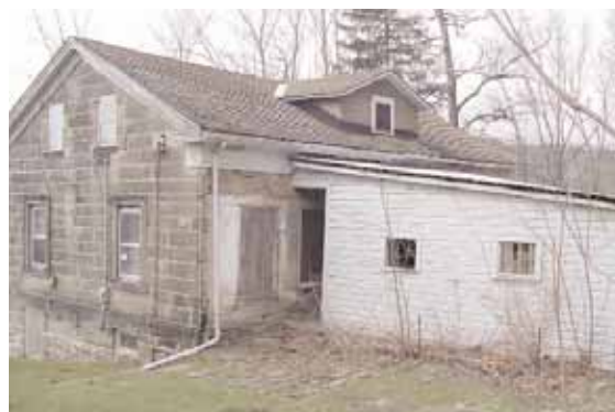
The back of the Gleeson home and carport addition, before rehabilitation. Spring 2001. NPS Photo.
