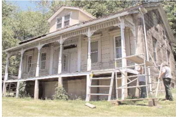
Workers begin to set up scaffolding at the front of the house to begin dismantling the front porch in early June 2005. NPS Photo.
