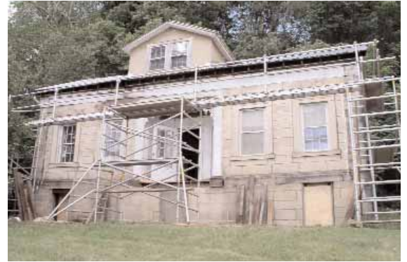
Front porch removed from the front of the house. June, 2005. NPS Photo.
