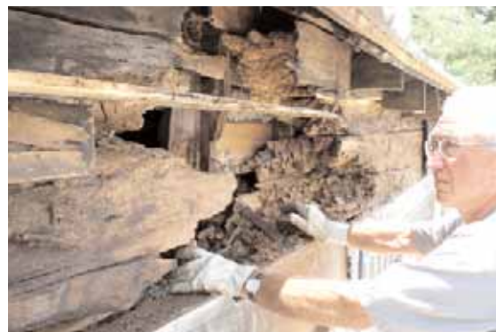
Extensive water damage to two large roof beams on top of the front wall. June 2005. NPS Photo.
