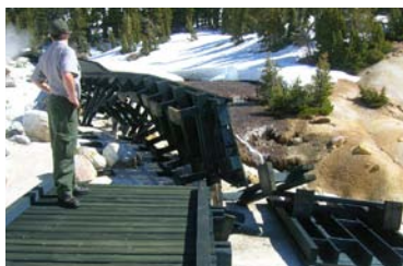
A park employee assesses damage to the pyrite pool boardwalk section.
