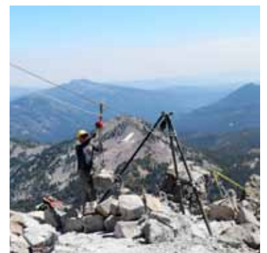
A pulley system allowed for the relocation of large stones deposited by helicopter in 2010.
