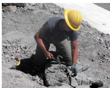
A trail crew member shapes stone for placement in a dry stone wall.
