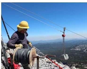
A pulley system allowed for the relocation of large stones deposited by helicopter in 2010.
