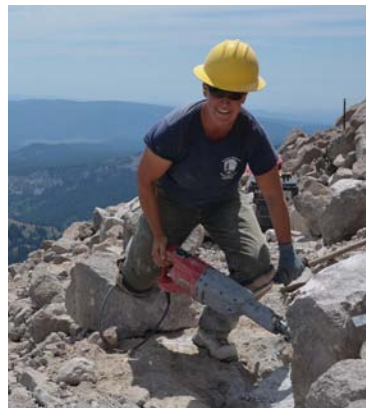
A member of the park trail crew prepares stone for placement in a retaining wall.
