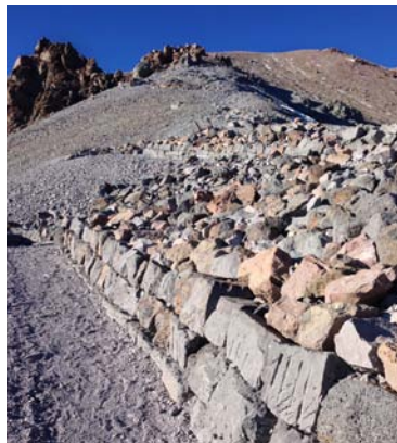
A retaining wall on the middle section of the trail reduces erosion and helps maintain trail width and prevent switchback cutting.
