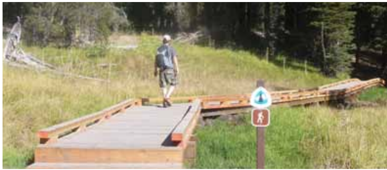
A hiker crosses a new section of boardwalk on the Pacific Crest Trail
