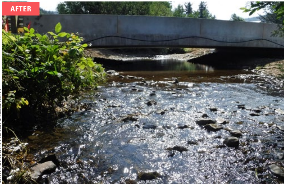
The Salmon SuperHwy partnership placed a bridge over Jewel Creek to replace three undersized culverts, restoring aquatic connectivity and improving transportation safety.
