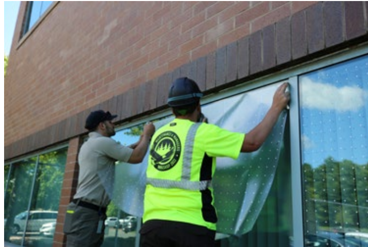
Maintenance professionals install bird-friendly materials to the windows of the Northeast Regional Office in Hadley, Mass. (PHOTO BY LEAH RILEY/USFWS)
