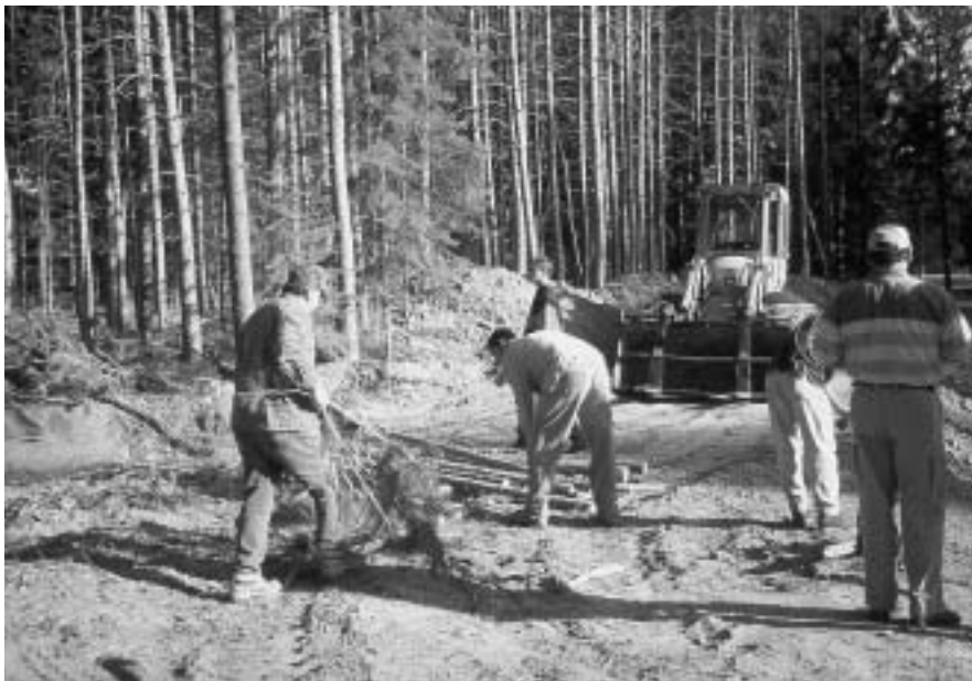
Volunteers from the Michigan United Conservation Club, Montmorency County Conservation Club and Thunder Bay River Watershed Restoration Committee assist Alpena FRO and other partners in bank stabilization at a bank erosion site on the Thunder Bay River in northeastern Michigan.
