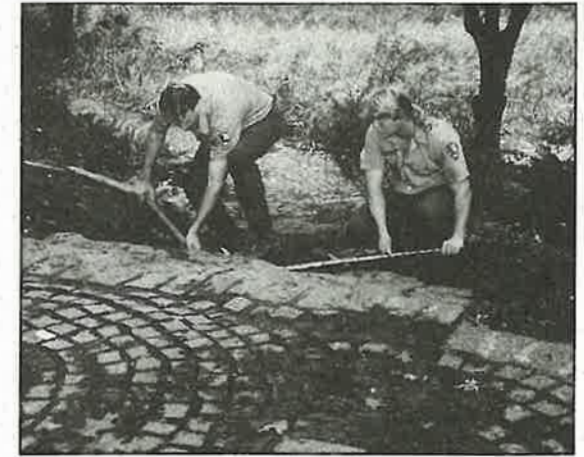
Landscape rehabilitation work at Minute Man National Historical Park by a multi-park preservation maintenance
