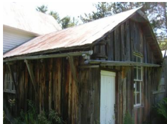
Treat rain-water system 2007
