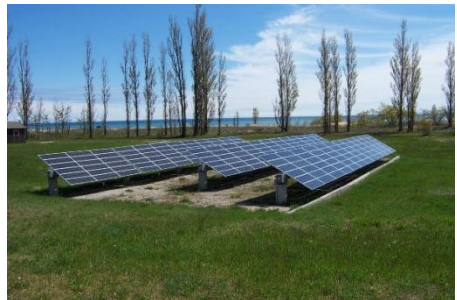
Photovoltaic array supplies power to the island.
