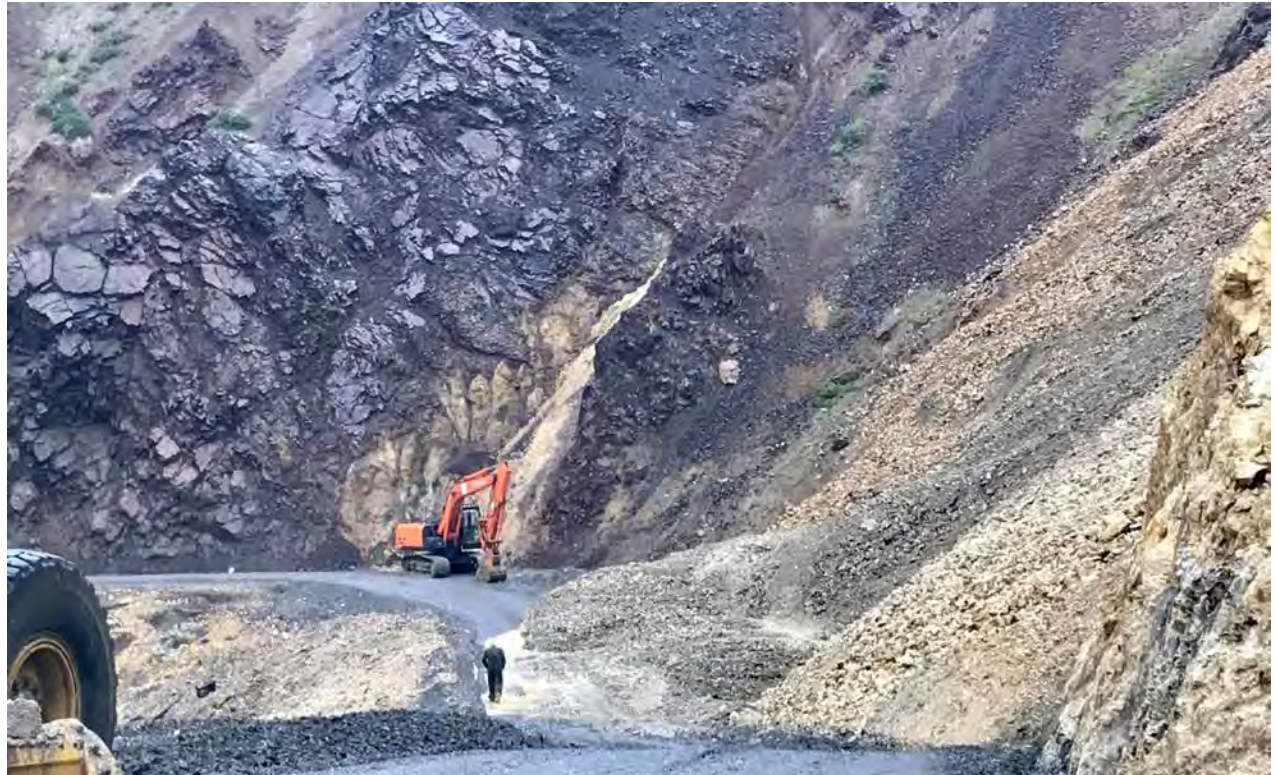
The Pretty Rocks landslide in 2019 after a heavy rain. NPS/WEEBEE ASCHENBRENNER
