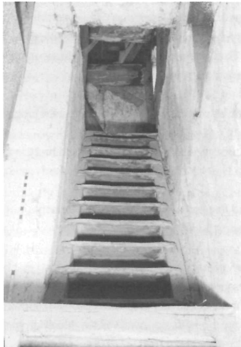
FIGURE 4 View of Stair from Third to Fourth Floor in the Cloisters, Saal, Ephrata, Lancaster County, Pennsylvania. HABS PA,36-EPH,1B-33, John O. Brostrup, Photographer, November 1936. (Courtesy of the Historic American Buildings Survey, National Park Service)
