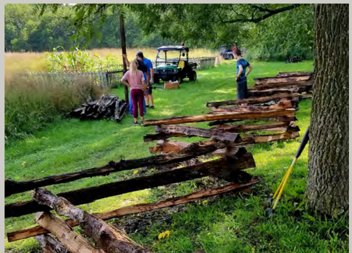
Gene Long and volunteers repair a split rail fence at GWCA (NPS).
