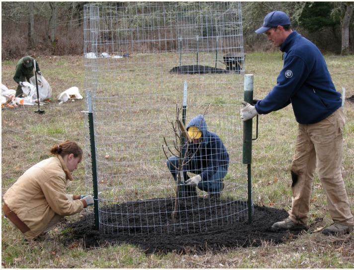
Construction of deer fencing around historic orchard tree replacement plantings at San Juan Island National Historical Park (NPS).
