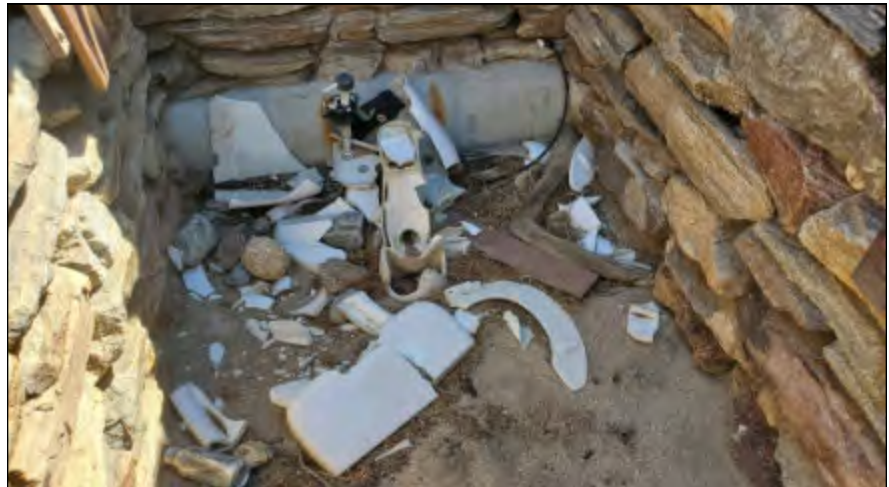
Borrego Palm Canyon campground facilities damaged by flood in 2004, still not repaired
