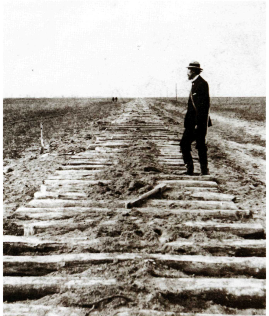
Monotonous flatlands extending to the horizon—and even beyond: Union Pacific construction on the transcontinental railroad in 1866.
