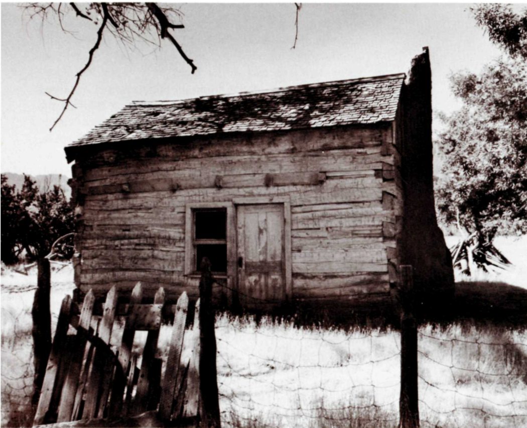
This log cabin in the ghost town of Grafton, near Zion National Park, embodies traditional half-dovetail corner notching and gable-end chimney; the chimney, however, is a papier-mâché fake added for use in the movie "Butch Cassidy and the Sundance Kid." The window directly adjoining the front door is a distinctive element of Utah cabins, including one preserved in Temple Square, Salt Lake City.
