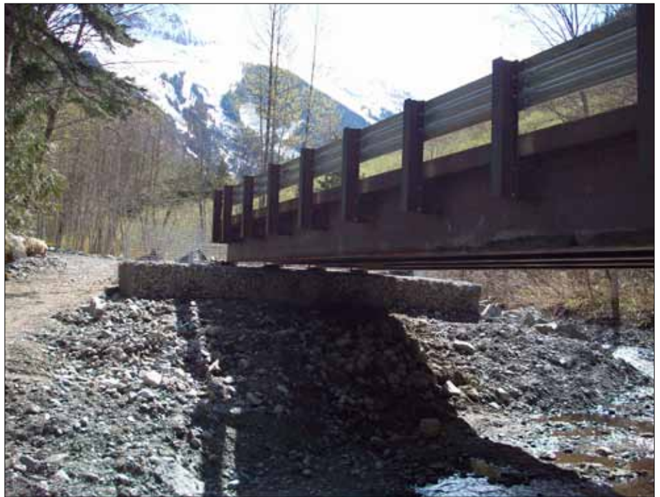
TOP: Flood damage in 2006 resulted in the closure of popular Cascade River road a few miles from its terminus.
