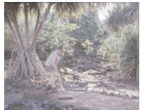
Installation of new stabilized walk surface. Pu'uhonua o Honaunau National Historical Park. Photo courtesy Peggy Nelson, NPS
