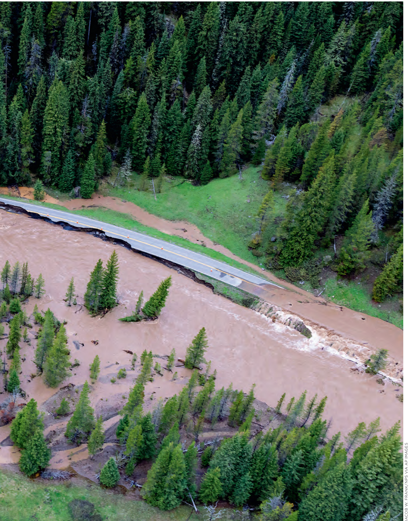
PHOTO: JUNE FLOOD WATERS RAVAGED THE NORTH ENTRANCE ROAD AND OTHER PARTS OF YELLOWSTONE NATIONAL PARK, MONTANA.
