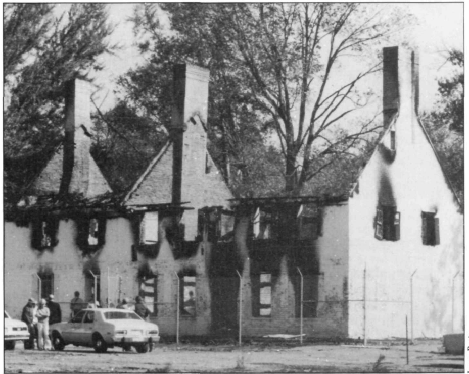
Arsonists succeeded in totally destroying historic Marshall Hall, Maryland, last October 16. The Park Service-owned mansion was 256 years old—
