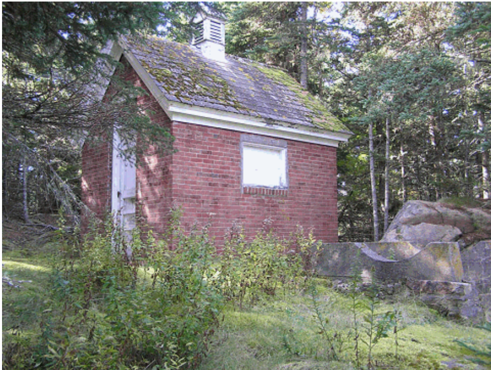
Figure 24. View of the ca.1895 oil house, looking west. The concrete cradles once held large tanks. (OCLP 2008)
