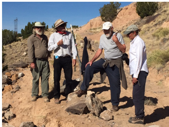
La Bajada (New Mexico) roadbed stabilization. Jake Barrow, Principal Investigator for Cornerstones Community Partnerships (second from left) conferring with USFS representatives and stonemasons.
