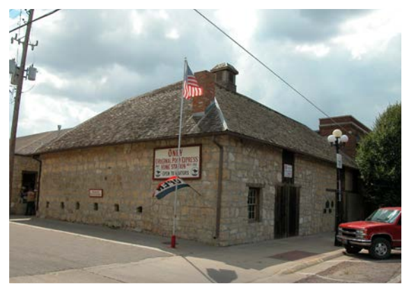
Staff with NPS's Vanishing Treasures Program worked with local partners on a preservation plan and structural assessment for the Marysville (Kansas) Pony Express barn.
