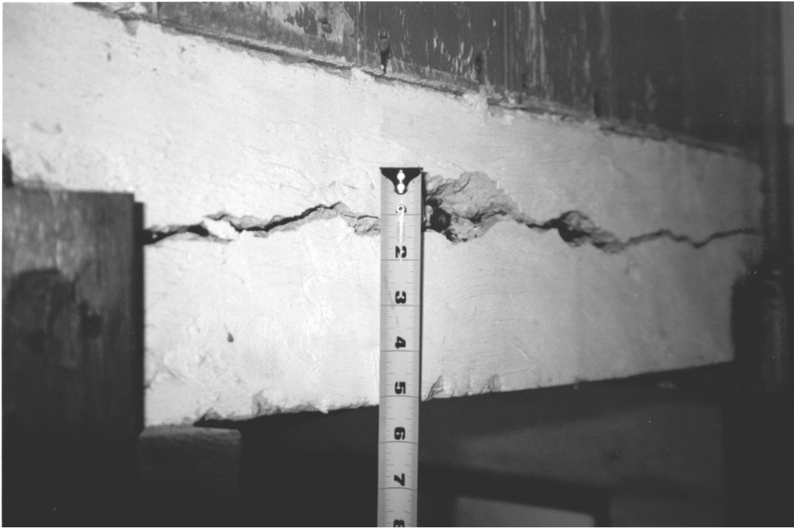
The crack at the first floor slab edge of the tower stair needs to be repaired or the slab edge must be supported by other means. Photograph 1999, McMullan & Associates
