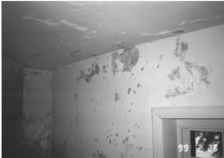
View of damaged plaster in tower, typical of damaged plaster throughout the building. Photograph 1999, architrave p.c., architects.
