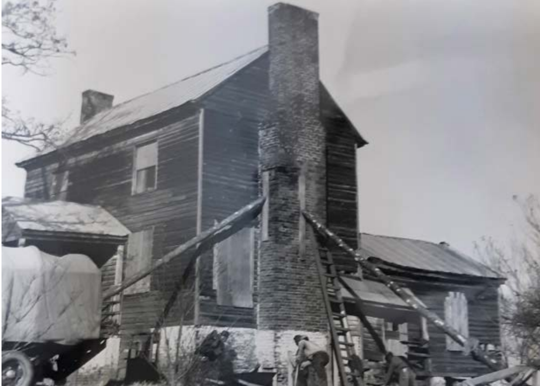
Figure 17. CCC enrollees stabilizing the Peers House south chimney as an example of jobs completed -after the McLean House reconstruction was delayed. SR, November 1941.
