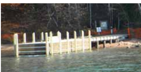
The rebuilt dock at Basswood Island is one of two new docks reopening this summer.
