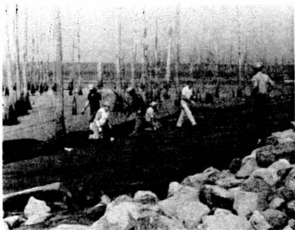
Placing filter cloth on Hurricane Mound in preparation for placing riprap, Sardis Lake, MS.
