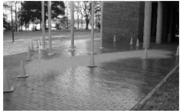
For the month of December slippery pavement, long-term power outages, and dangerous tree limbs were the norm for the Post.
