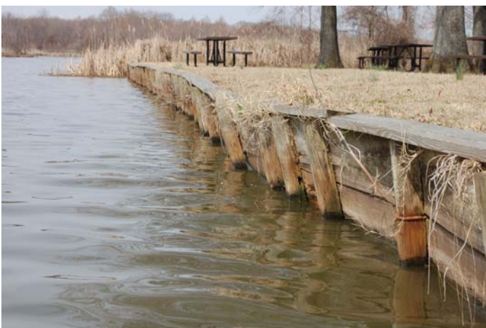
Old retaining wall was rapidly deteriorating.
