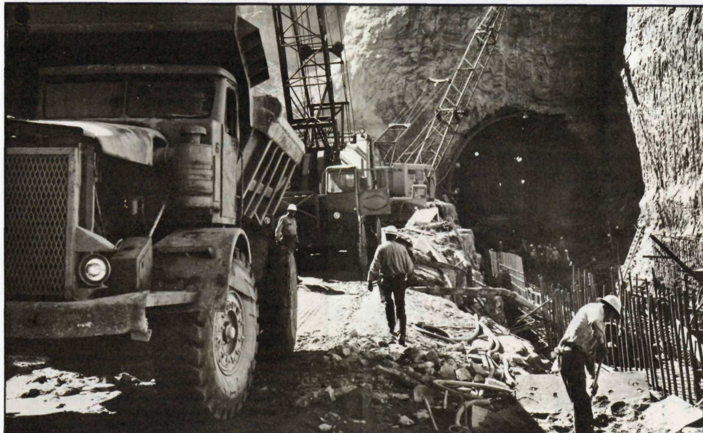
Construction operations in stilling basin in front of outlets to 1,700-foot-long spillway tunnel excavated through solid rock canyon wall
