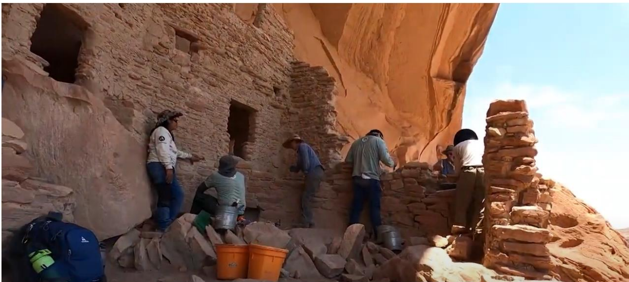
Figure 4: An Ancestral Lands Corp crew works to stabilize the River House ruin in Bears Ears NM.
