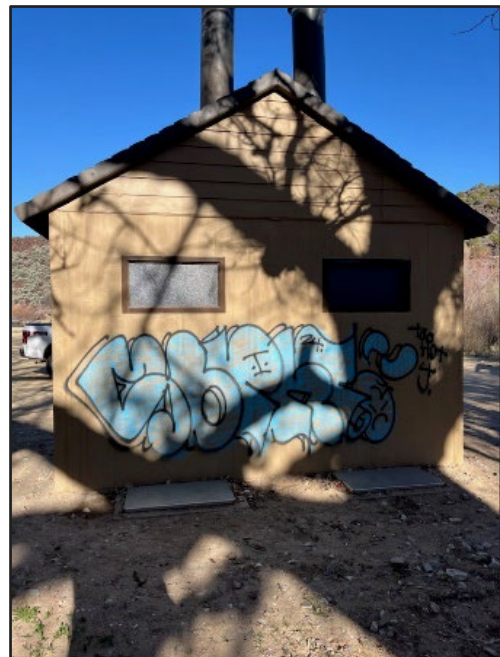
Graffiti recently removed from Quartzite pullout
