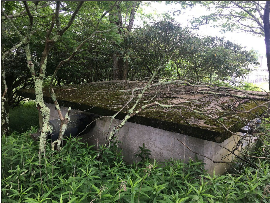
Fig 8-20. Fallen branches littering Pump House roof, facing southwest (2021)
