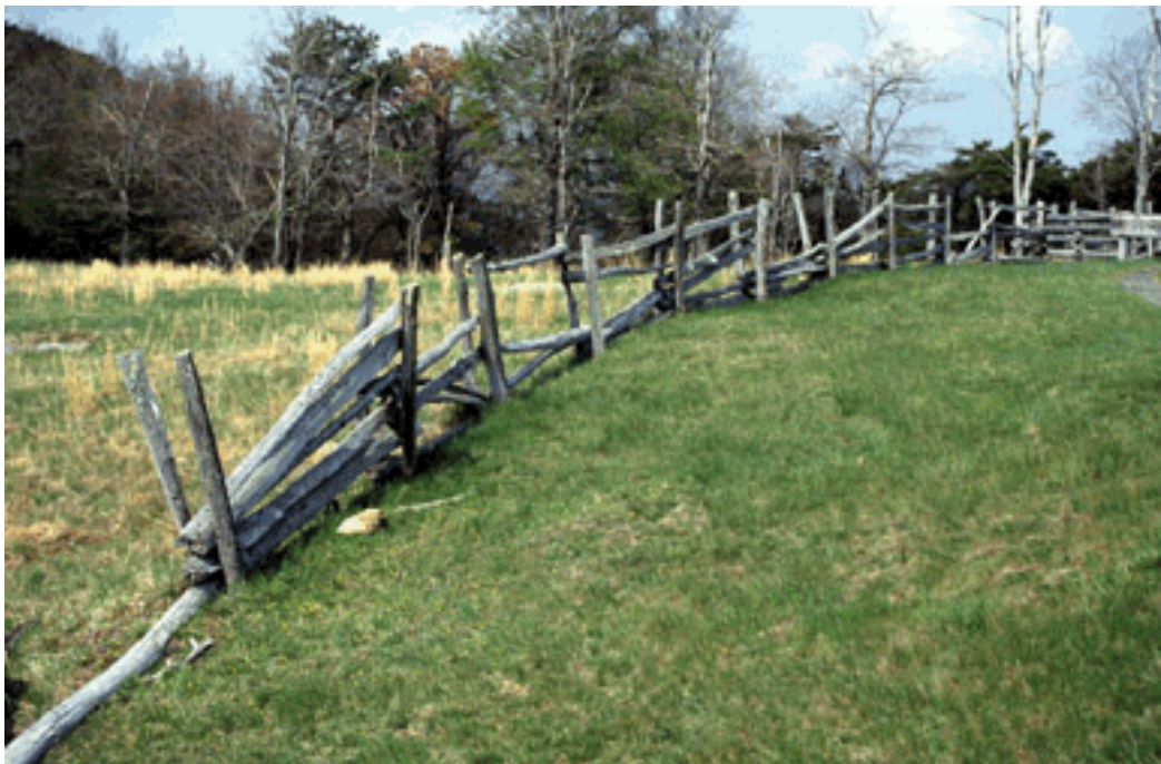
Fence in disrepair (2002)
