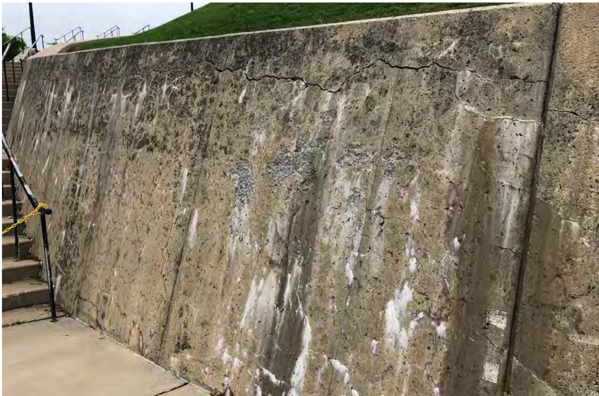
(top and bottom) Figures 3-36 and 3-37: Sample conditions of retaining walls at entrances, stairs, and ramps
