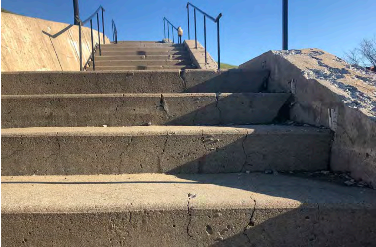
(top left and right) Figures 3-30 and 3-31: Closed stairway to the southwest and open stairway at the northwest (bottom) Figure 3-32: Western stairs showing cracking and spalling on the steps and walls
