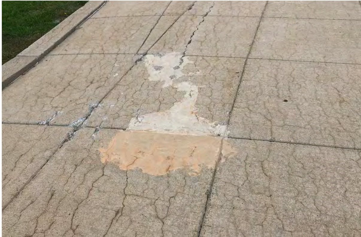
(top left and right) Figures 3-25 and 3-26: Sample conditions of walkways showing spalling and puddling expanding from expansion joints
