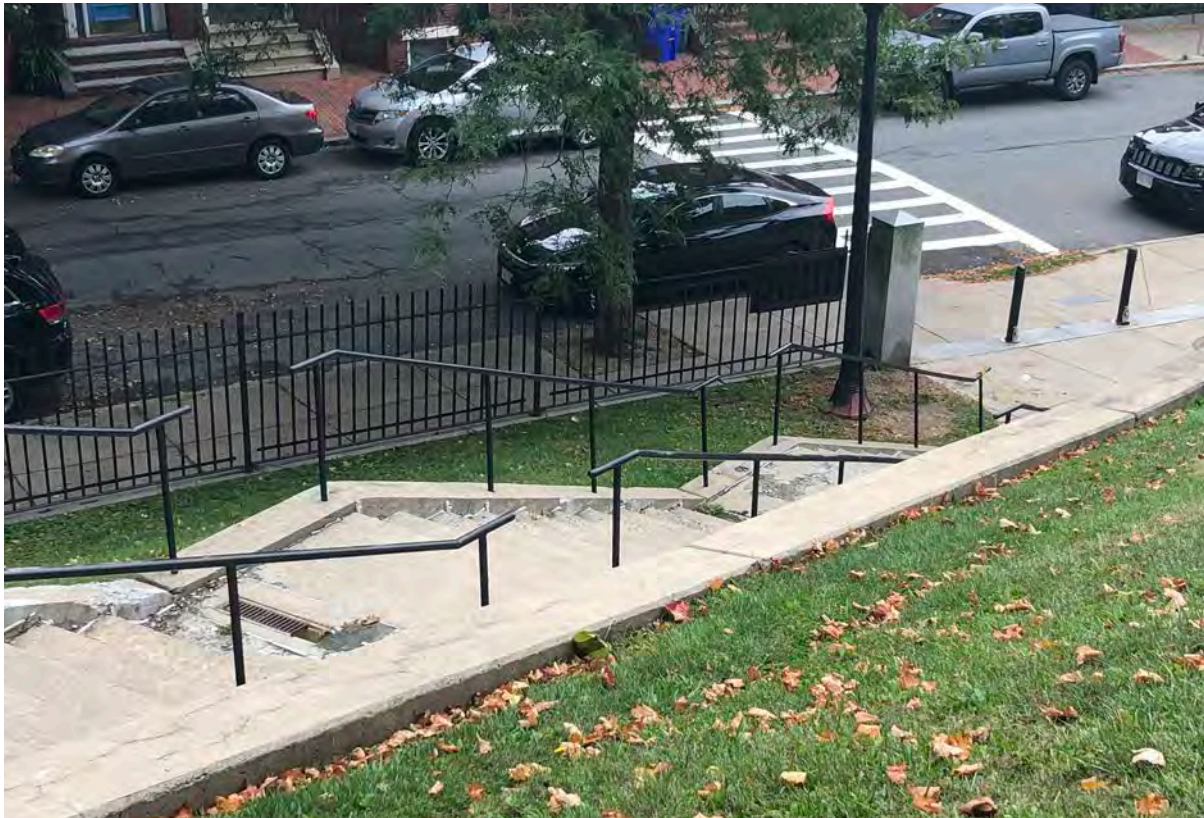
(top) Figure 3-40: Sample ramp handrail with rail segments missing
