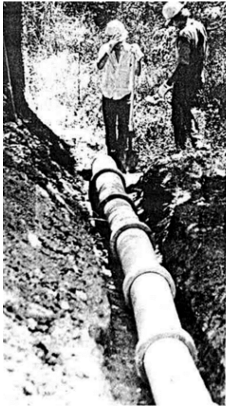
Youth Conservation Corps workers began digging a drainage ditch at Booker T. Washington National Monument last week. The project is one of 22 the corps hopes to complete by the end of the summer.
