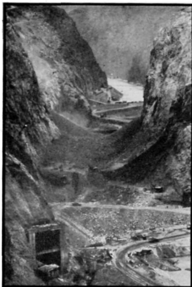
Debris in Canyon, Following Excavation on Canyon Walls
