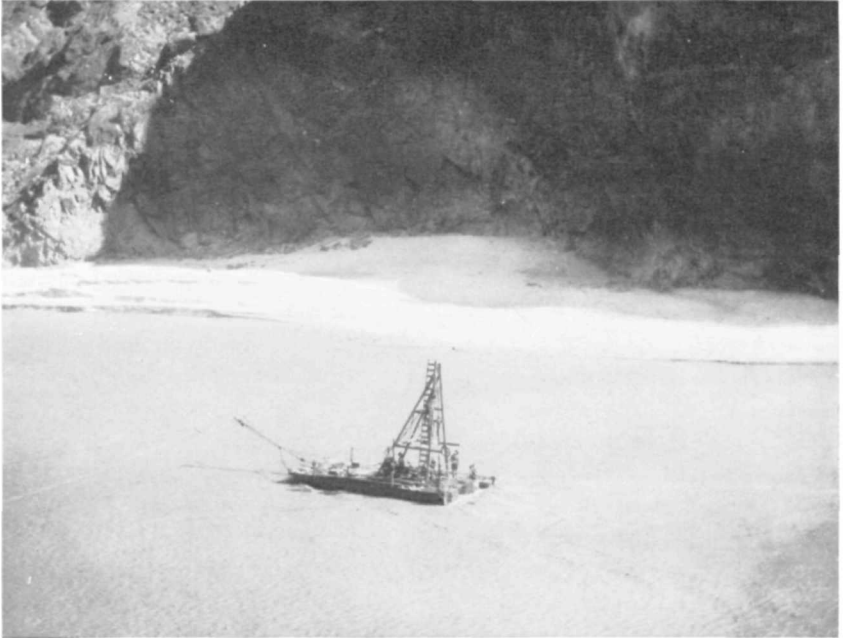
Drill barge exploring Hole 1-4, testing thickness of lava in the Colorado River bed
