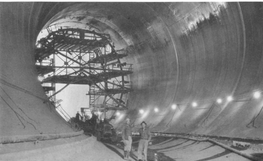
A big hole for the river to flow through—one of the diversion tunnels
