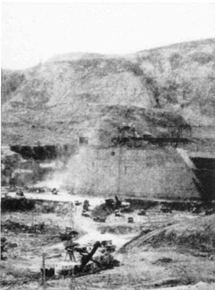
Removing from the old channel of the diverted river deep beds of clay deposited during the last Ice Age
