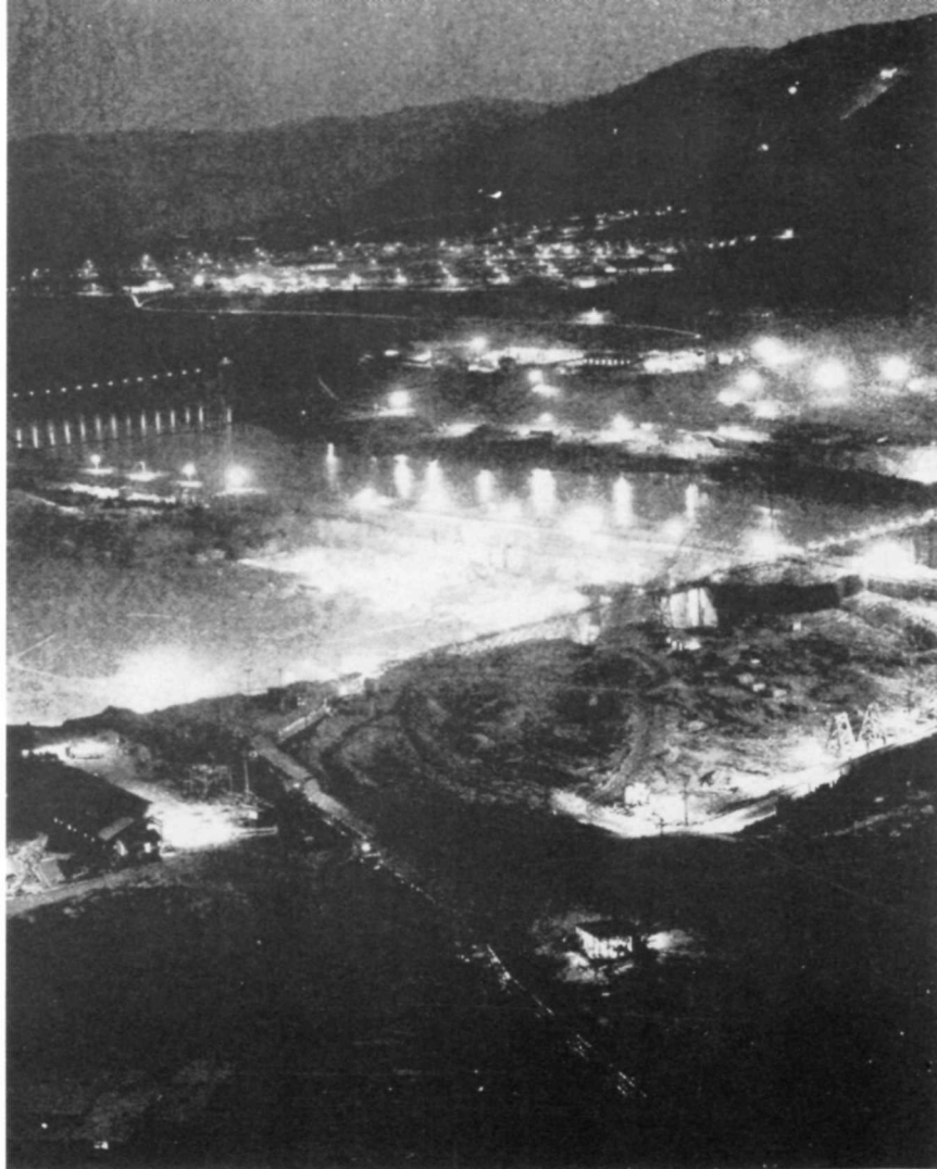
Above: Under powerful lights covering an area 3 miles long, work on the base of the dam went on day and night without interruption Left: 127 miles of heavy steel sheet piling was driven in the west cofferdam by powerful steam hammers
