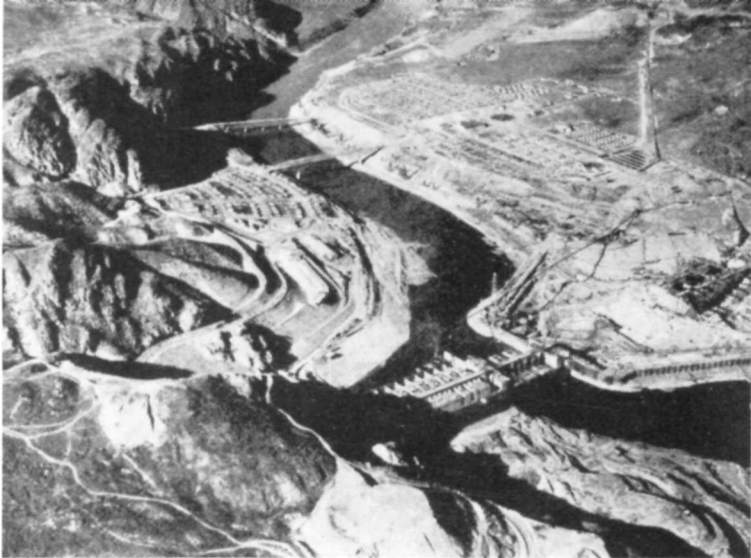
Aerial view of Grand Coulee Dam, looking northeast over the construction area, the Government town, Coulee Dam (left), and the contractor's town, Mason City, in April 1937. (15th Photo. Sec., U. S. Army)
