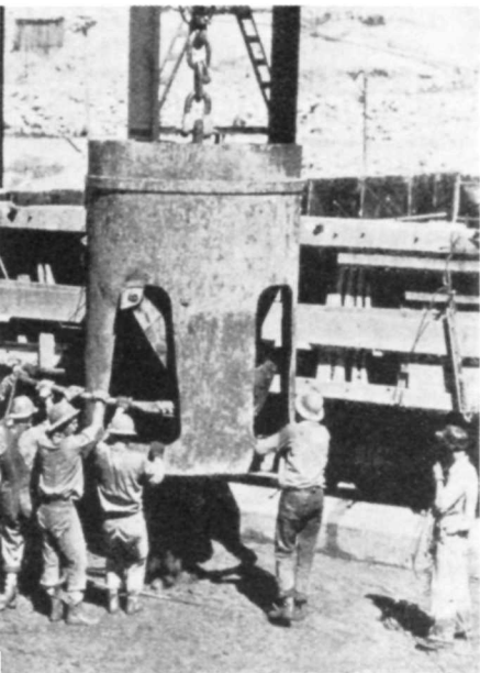
Eight-ton batches of concrete are handled by huge overhead cranes, directed by telephone-signalmen "on location"
