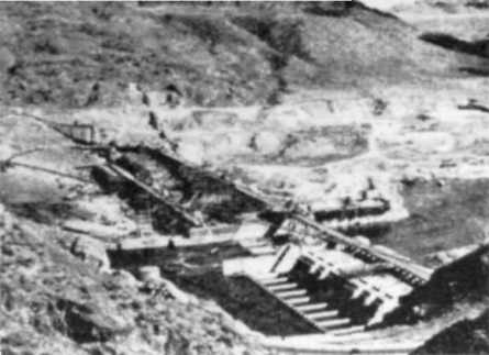
Columbia River diverted through base of dam built inside west cofferdam. Excavation under way in old channel, 1937
