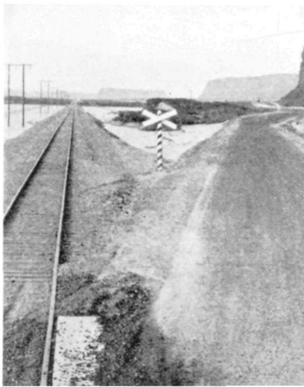
Left: Rockmen drilled, blasted, and barred down thousands of tons of weathered and loose rock from abutment areas
