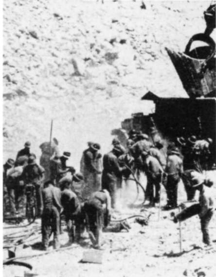
Jackhammers and dynamite moved a million yards of rock to make a firm, clean footing for the dam
