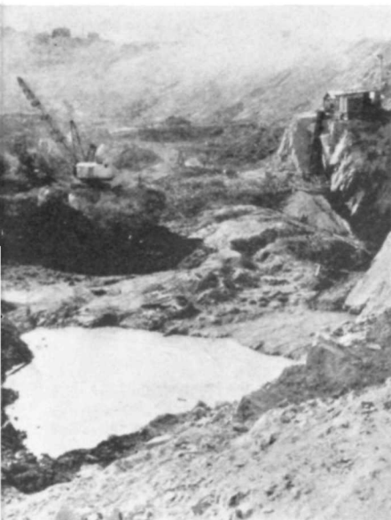
Six miles of refrigerating pipe were driven into the toe of a 200,000-yard mass of moving clay
