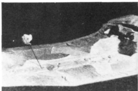
Three deep gorges and numerous minor irregularities were found at the bottom of the 18-million-yard excavation
