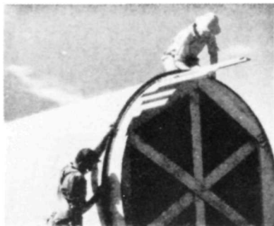
Two and a half miles of cylindrical forms will be required for the 8\frac{1}{2} -foot outlet tunnels
