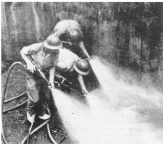
Four-yard batches of concrete, in huge steel buckets, were lowered into the forms by long-arm cranes. After at least 3 days, each lift was scrupulously cleaned with sandblast, air, and water before another was laid on it
