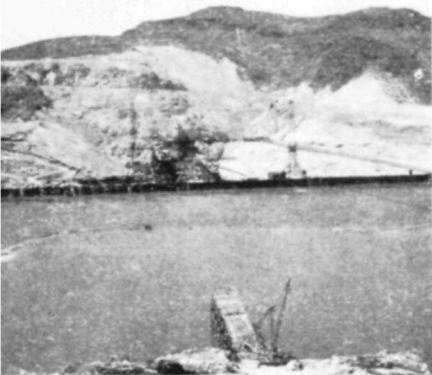
High water flooded the low east cofferdam in 1935, but the west cofferdam kept a 60-acre working area dry
