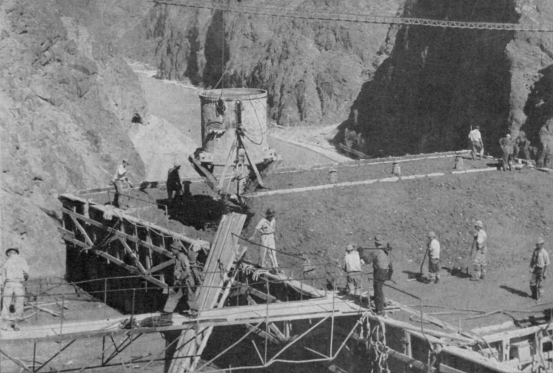
Boulder Canyon. Eight cubic yard capacity bucket discharging load into dam forms at upstream face of dam.
