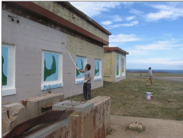
AmeriCorps Cape Cod member Ben Fairbank applies a fresh coat of paint to one of the buildings.
