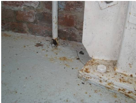
Figure C-22 Corroded connecting rod at Watch Room floor plate.
