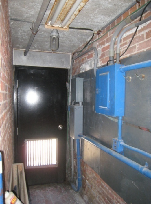
Figure C-59 Currently operational electrical panels on west wall of entrance passage.
