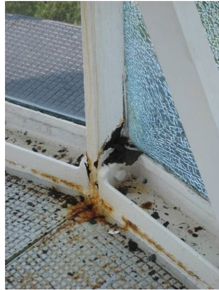
Figure C-98 Deteriorated iron framing.
