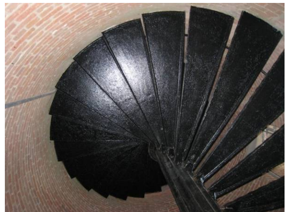
Figure C-41 Typical Spiral Staircase section as found from Second Floor to Seventh Floor.
