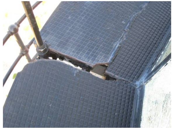
Figure C-23 Broken floor plates of Lantern Gallery.
