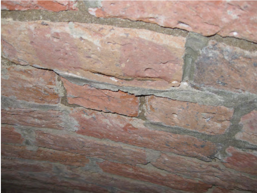
Figure 20. Cape Lookout Lighthouse, September 2008. An area where inappropriate Portland cement based re-pointing mortar has caused the original brick to spall and the original mortar to deteriorate. Photograph by author.
