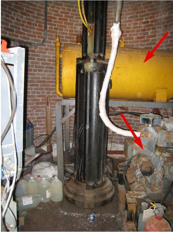
Figure C-13 Center column on sandstone pedestal, abandoned emergency generator and fuel tank nearby.
