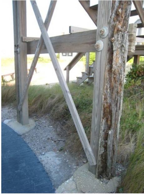
Figure C-34 Two earlier but twentieth-century and severely deteriorated wood posts and one cross beam
