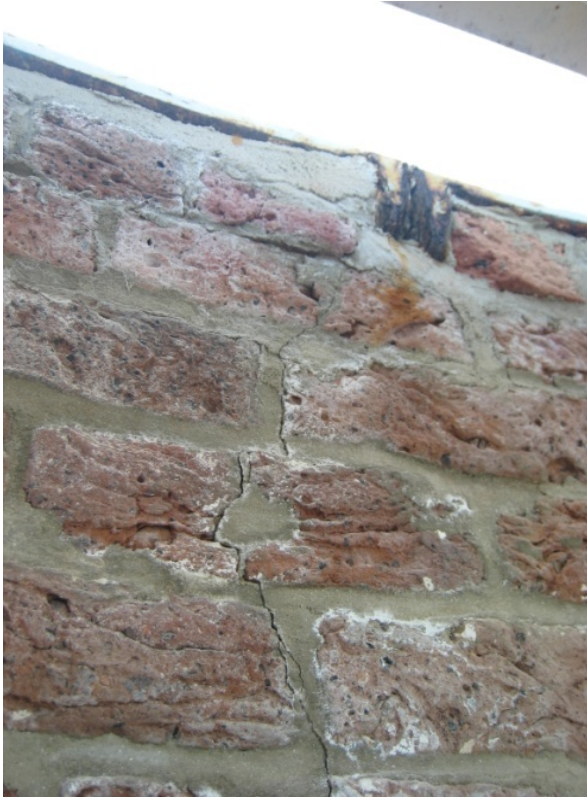
Figure C-105 Through-wall cracks in masonry at top of Tower.
