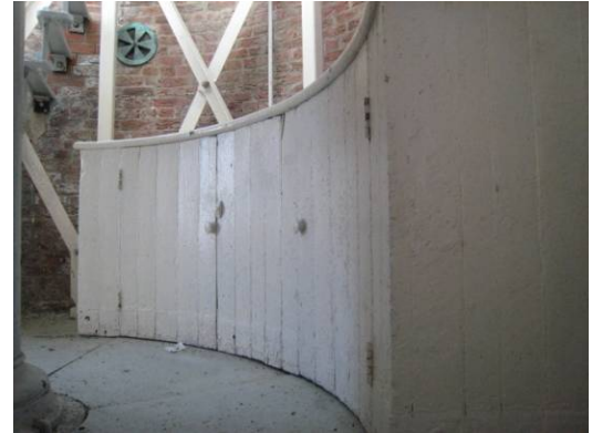
Figure C-91 Two-door cabinet in Eighth Floor Watch Room.
