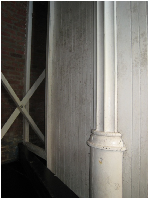
Figure C-77 1914 board wall and doorway at Seventh Floor landing. Note 1989 steel reinforcement added at masonry perimeter.
