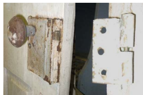
Figure C-78 Salvaged four-panel door; detail images of rim lock with sheet metal doorknob and two-knuckle brass hinge. (North Carolina Maritime Museum Collection)
