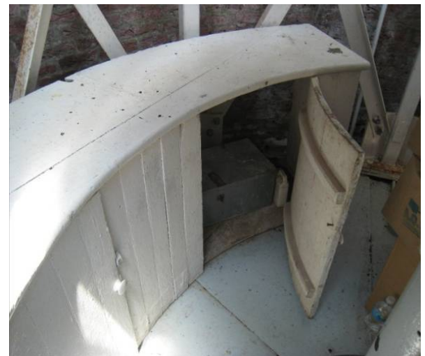
Figure C-51 Watch Room cabinet.
