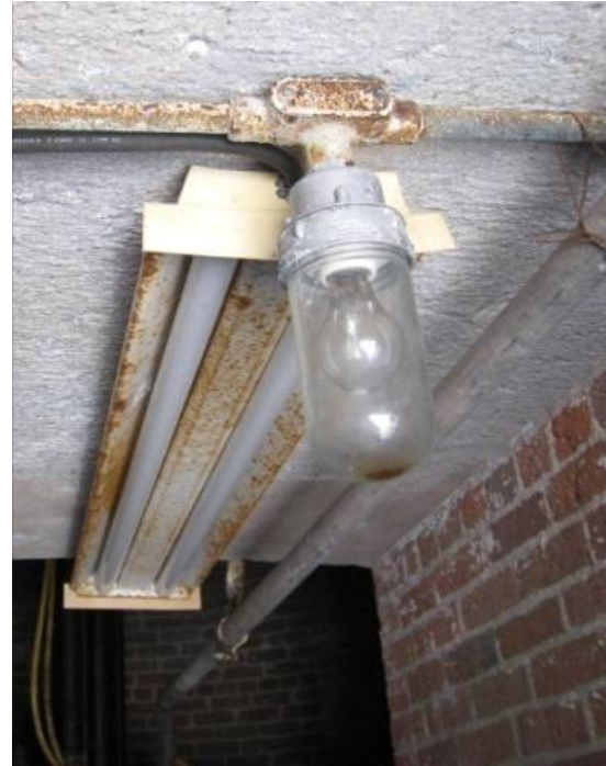
Figure C-57 Metal electrical conduit with incandescent and fluorescent light fixtures.
