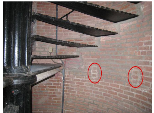
Figure C-68 Two masonry patches presumably associated with the 1864 framing for temporary stairs.
