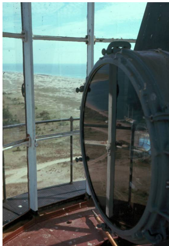
Figure C-53 1976-1981-era photograph showing red primer on lantern floor (CALO Coll.)
