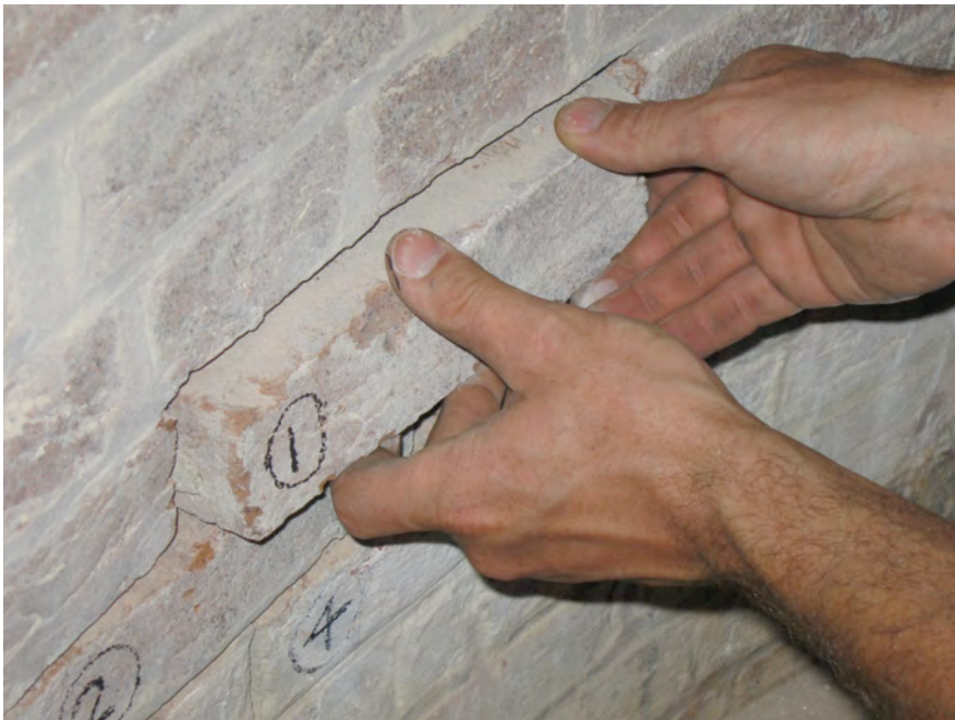
Figure 4. Cape Lookout Lighthouse, October 2008. Removal of a brick for laboratory testing. A total of five bricks were removed from the building. Photograph by author.
