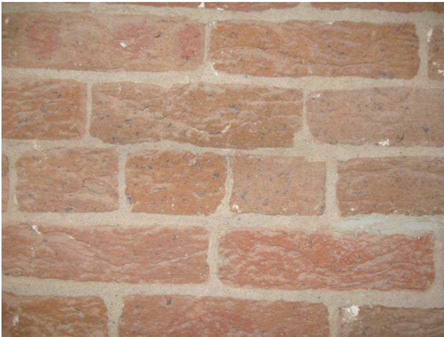
Figure 19. Cape Lookout Lighthouse, September 2008. Area of typical interior brickwork showing the brick's hand-pressed, low-fired quality and appearance. Photograph by author.
