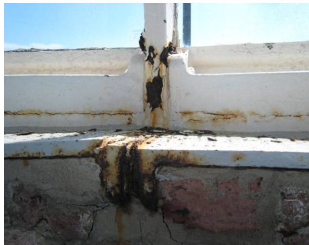
Figure C-104 Extensive corrosion of cast-iron framing.
