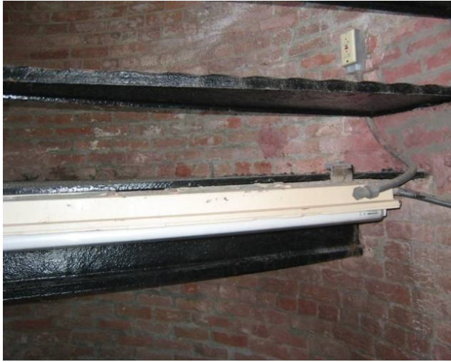
Figure C-19 Typical shop-type utility lighting at spiral stairs floor landing.
