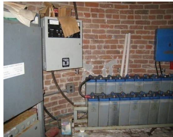
Figure C-58 Abandoned power controller and fuel cells.
