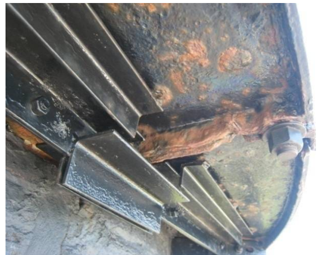
Figure C-106 Underside of Lantern Gallery reinforced in 1989.
