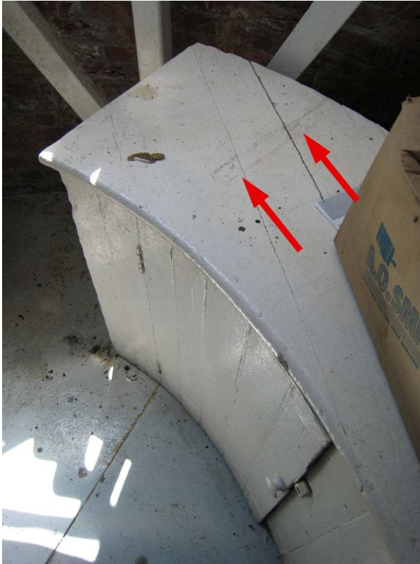
Figure C-93 Ghost marks of missing shelving supports.
