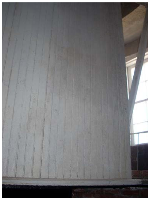
Figure 5 – Bracing Interrupting Partition Wall at Storage Area
