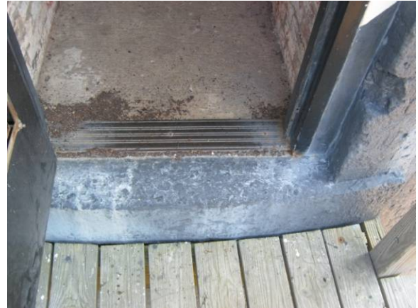
Figure C-40 Granite doors sill at Second Floor entrance. Note modern infill, door frame, and door.
