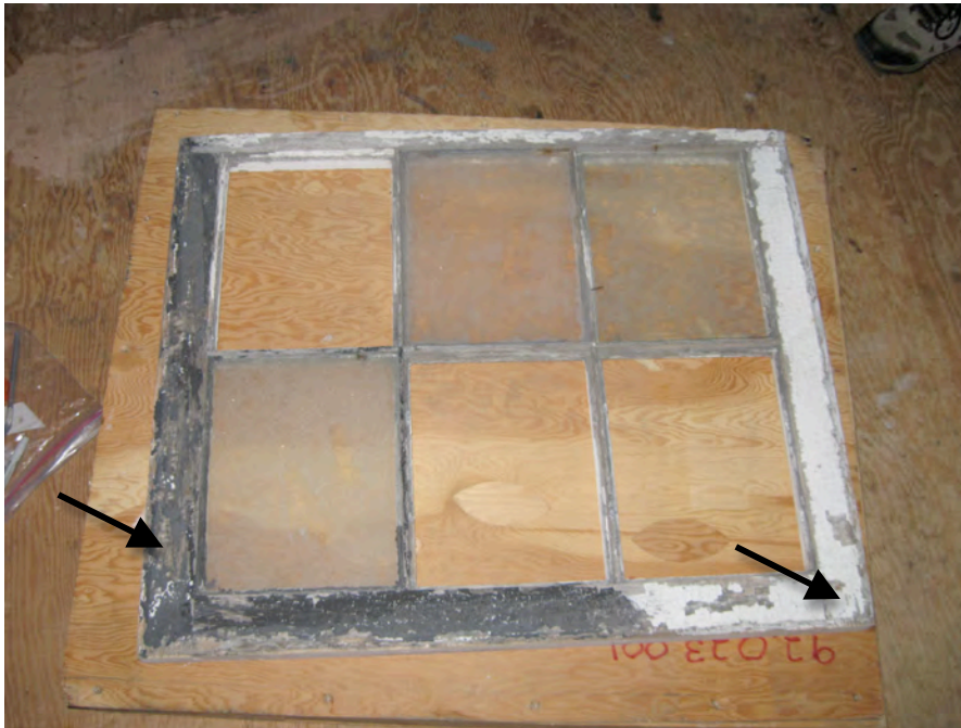
Figure 9. Cape Lookout Lighthouse, October 2008. A salvaged window sash currently located at the North Carolina Maritime Museum. Two samples were removed from the exterior face of the sash (arrows). Photograph by author.
