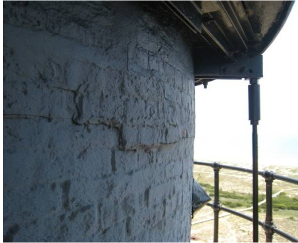
Figure C-107 Displaced masonry and supplemental tie rods.
