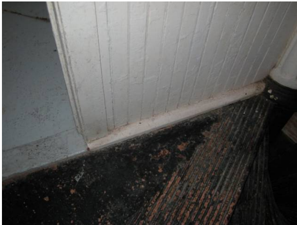
Figure C-80 Door threshold and board wall at Seventh Floor, the top landing of the spiral stairs.
