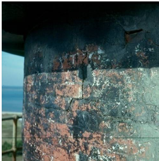
Figure C-12 A 1976-1981-era photograph of exterior masonry at Observaton Deck.
