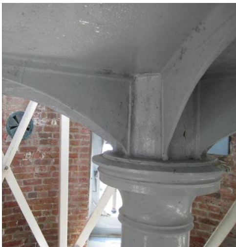
Figure C-88 Column and underside of cast-iron platform for beacon.
