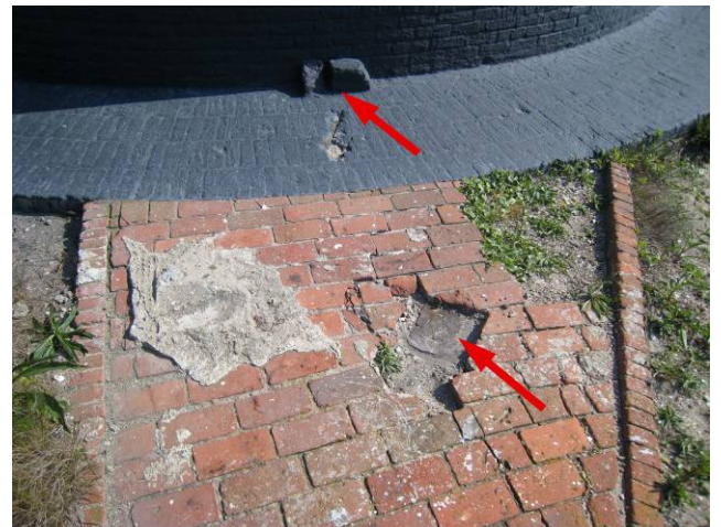
Figure C-33 Brick Apron at intersection with brick walk to Keeper's Quarters. Note post and stone base for previous stairs.
