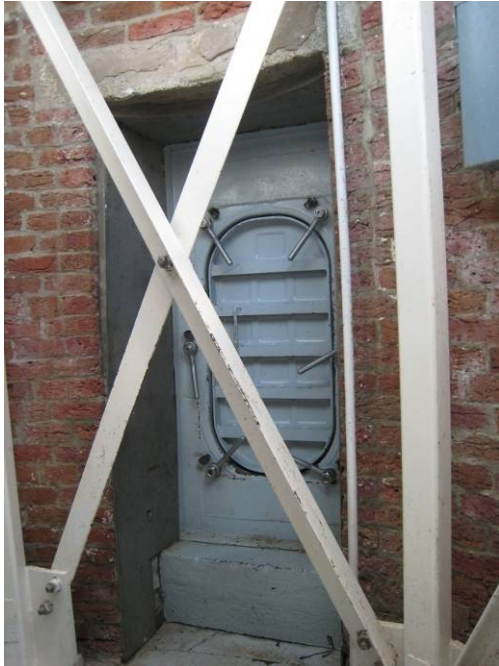
Figure C-87 Reinforcing steel added in 1989 partially blocks ship's hatch to Observation Deck.
