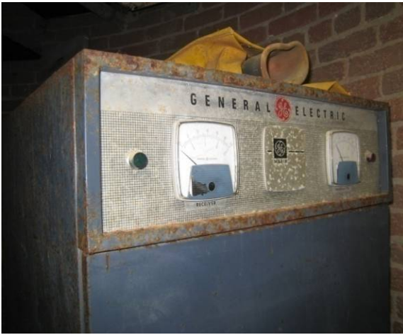
Figure C-63 Abandoned GE transmitter/receiver.
