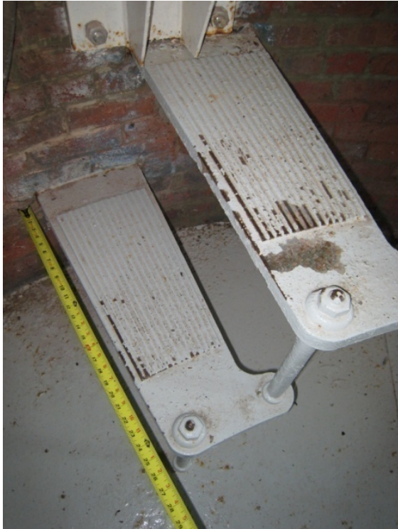
Figure C-82 Original cast-iron ship's ladder stairs connecting Seventh Floor Service Room to Eighth Floor Watch Room.
