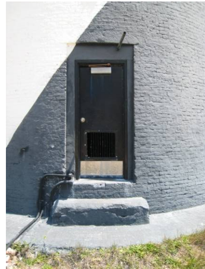
Figure C-28 Original masonry opening for First Floor doorway with modern infill and steel door.
