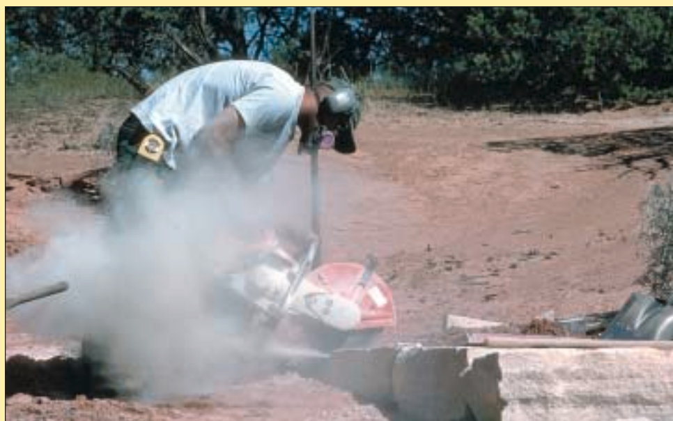
Reconstruction of the Mesa Arch Trail at the Island in the Sky.
