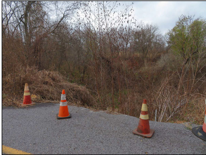
Fig 3.4. Embankment failure along the slope of Cane River west of LA-119 and west of the Store has compromised the road integrity. Heritage Landscapes.
