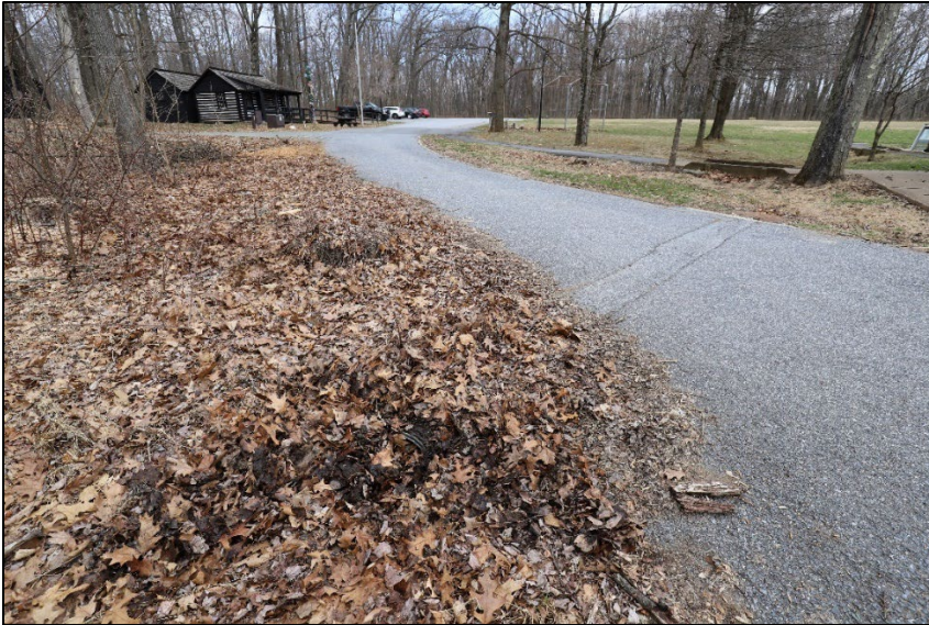
Fig 45: Culvert obscured by leaves, located west of the recreation hall. (NCR 2023)
