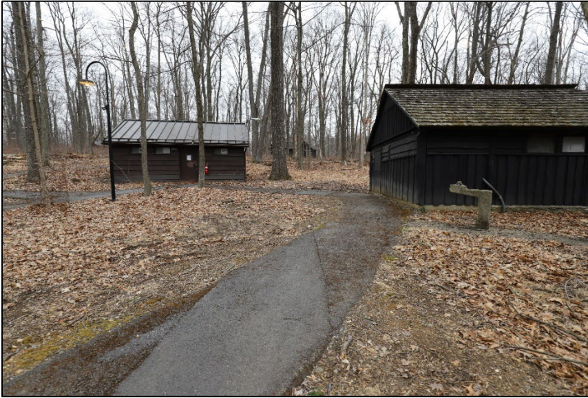
Fig 28: Asphalt paved pedestrian walkways impacted by recent utility work. (NCR 2023)
