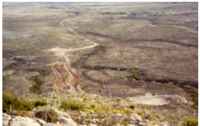
NEW WATER LINE – In this January 1999 photo, the new water pipeline and accompanying infrastructure can be easily seen from the escarpment edge near the Visitor Center. (NPS Photo by Stan Allison)
