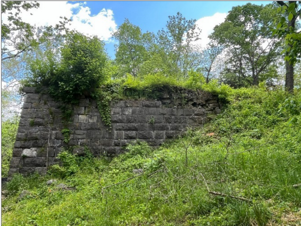
Old Valley Pike bridge abutment with woodland and other vegetation growing on and around it. This abutment, which is on NPS property, dates back to about the 1830s. Image Credit: NPS NRCA Program.
